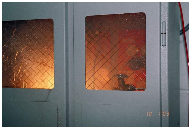
Fig. 16: Silane Leak at Outlet Connection, Pigtail Valve Has Automatically Closed
