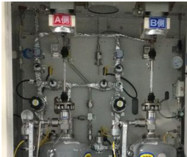
Fig. 21: Festo Valve Shutoff
