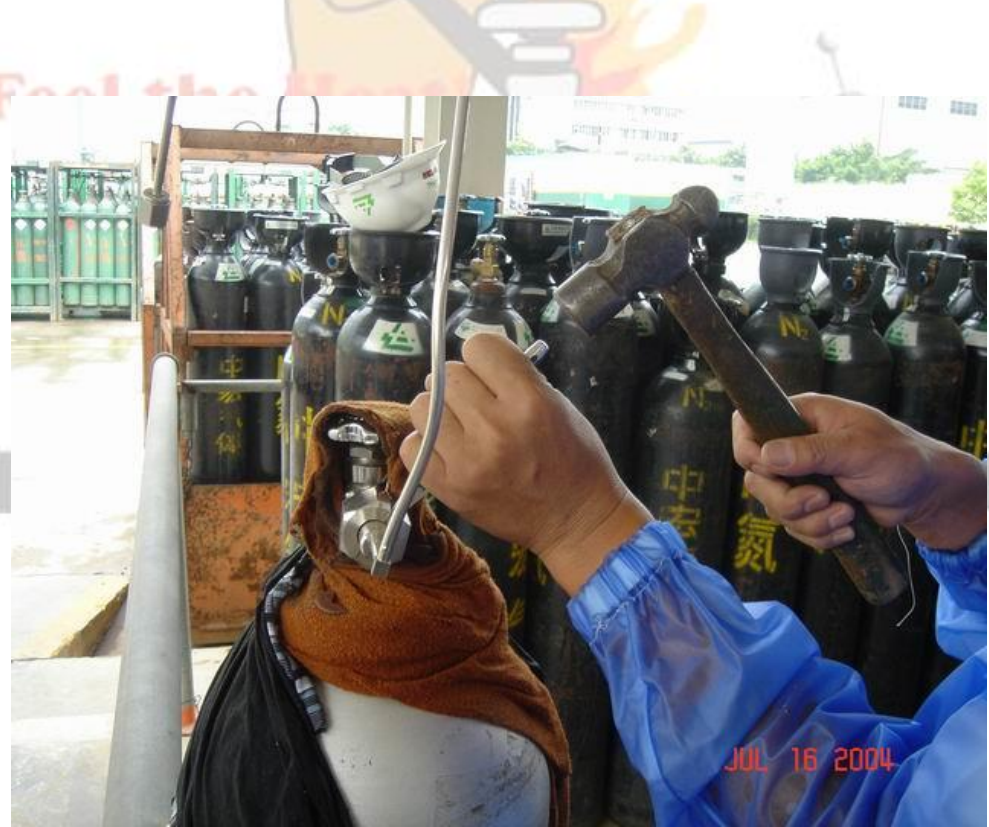
Splitting the nut with Chisel after cutting the nut with the grinder tool (but use gloves!).
