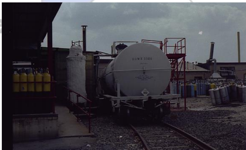
Fig. 2: Older HCl Railcar with Cooling Coil
