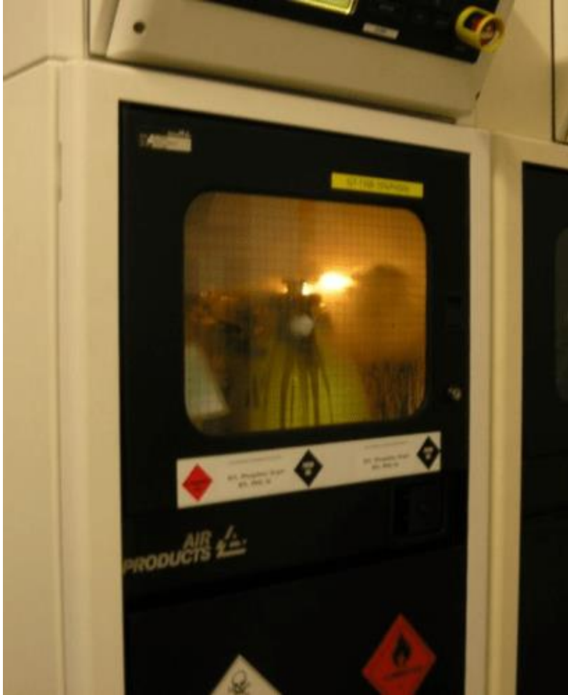
Figure 3 – Burning phosphine after autoignition from cylinder valve connection leak in a gas cabinet at a semiconductor facility. This cylinder contained 15% phosphine in argon gas.
